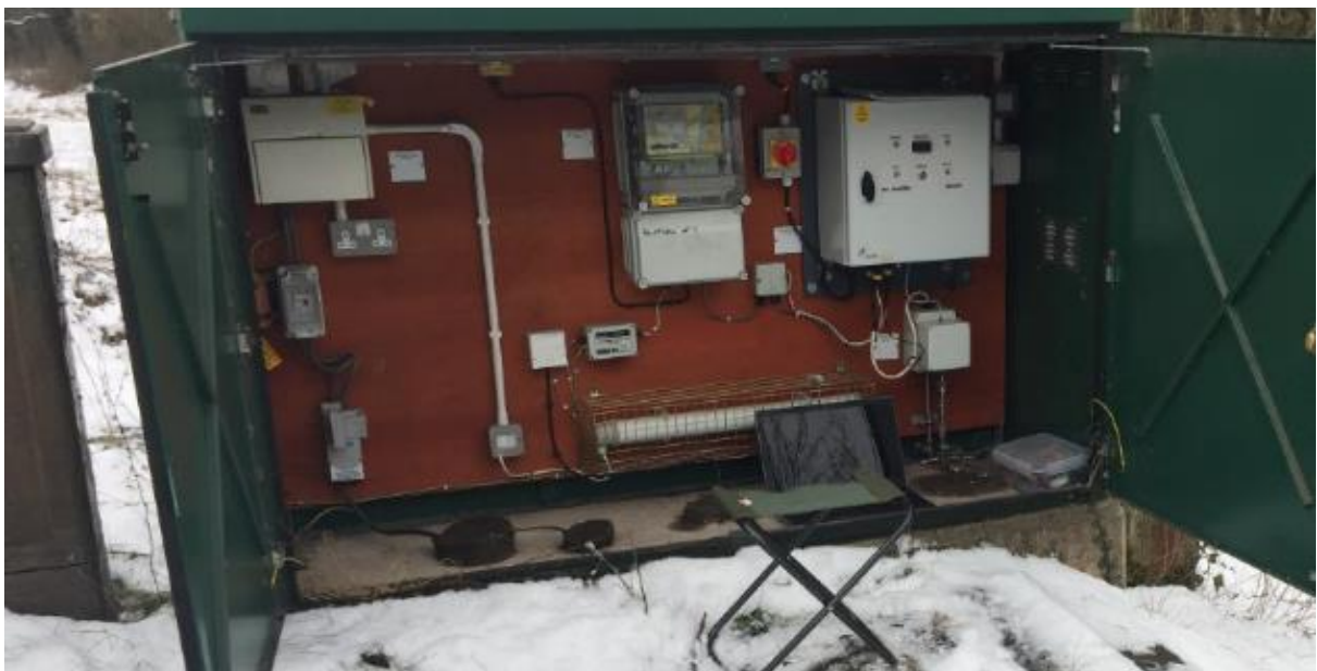
Unit installed in a cabinet. There are 6 of these cabinets on the industrial estate and include heating system, lighting protection and connection to the telemetry system.
