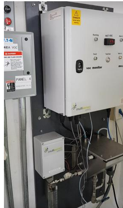
Photo showing the MS1200 installed in the Pump Station. The unit is connected to a SCADA system (Ethernet) using the Profibus Protocol (TCP / IP), which records the data and, in case of an accident, activates the alarms that shut off the suction pumps.
