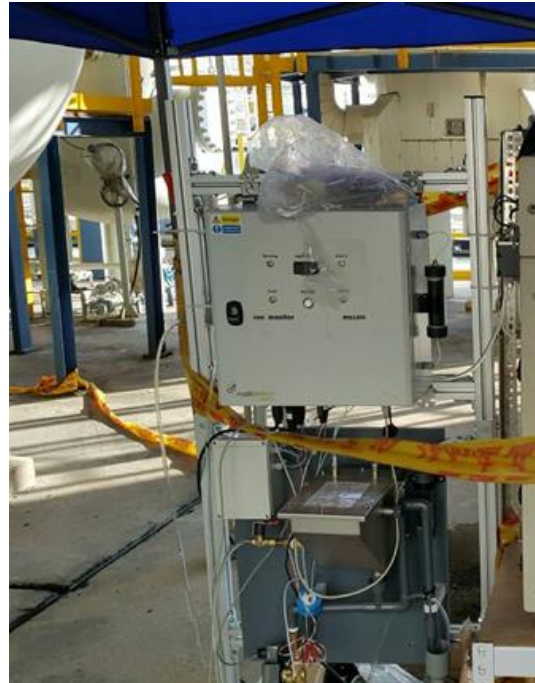
Photo showing the MS1200 in the petrochemical plant
