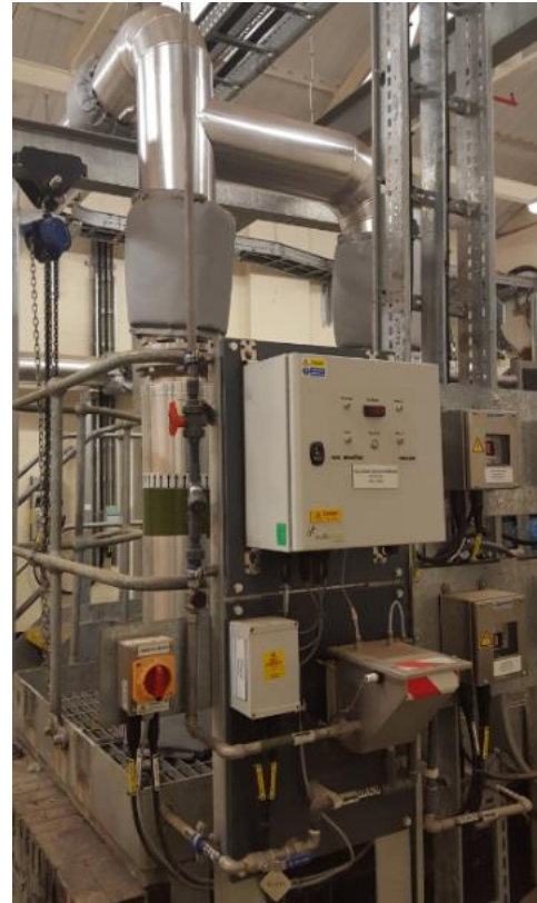
A picture of the unit installed in the factory.
