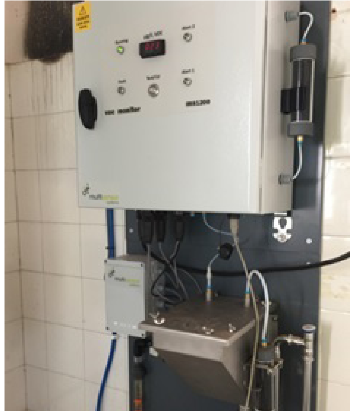
A picture of the unit installed in an outbuilding next to the borehole.
