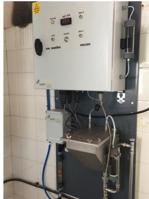
A picture of the unit installed in an outbuilding next to the borehole.
