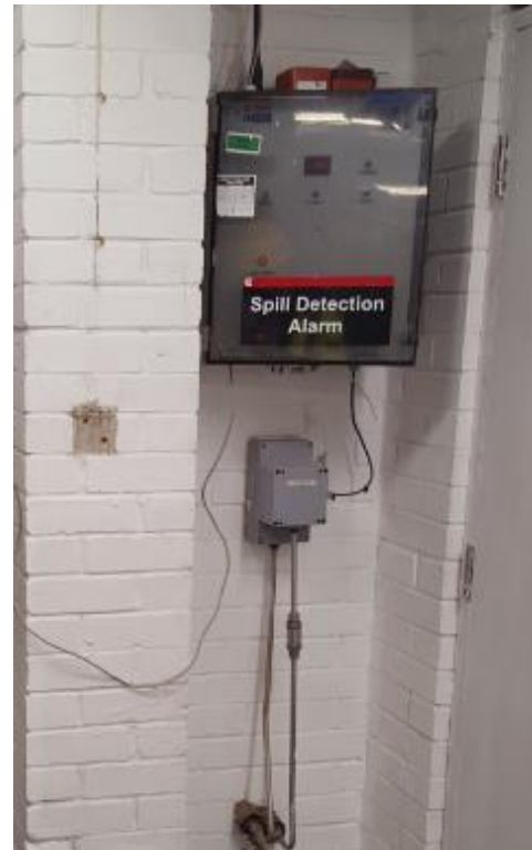
A picture of the unit installed in the manufacturing plant
