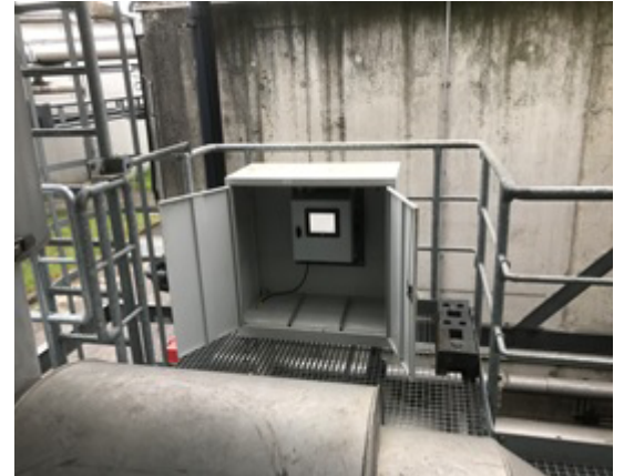
A picture of the unit installed in the cabinet for further weather protection
