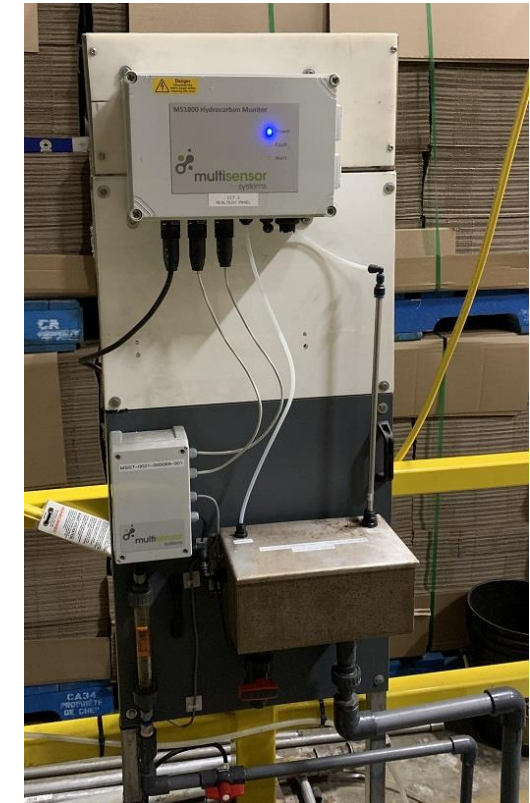
The MS1900 analyser installed close to the effluent.
